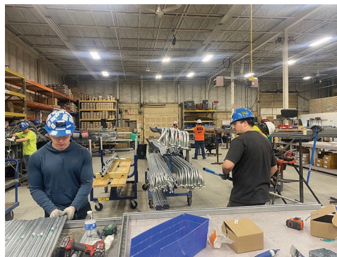
Prefabrication technology has several advantages: energy efficiency, minimal waste and inspection, efficient construction, work speed, safety, sustainability, and quality.
